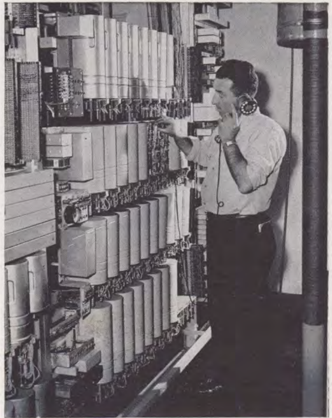
In Scituate, Rhode Island, Howard H. Chilton, Central Office Repairman, inspects the community dial office before the installation of additional equipment to take care of rural growth in that community.
