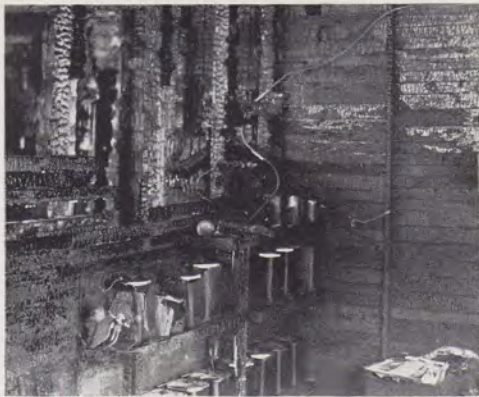
This picture shows what would have happened to the switchboard had not help arrived to move it. Shown are the charred walls and batteries in a corner of the office.
