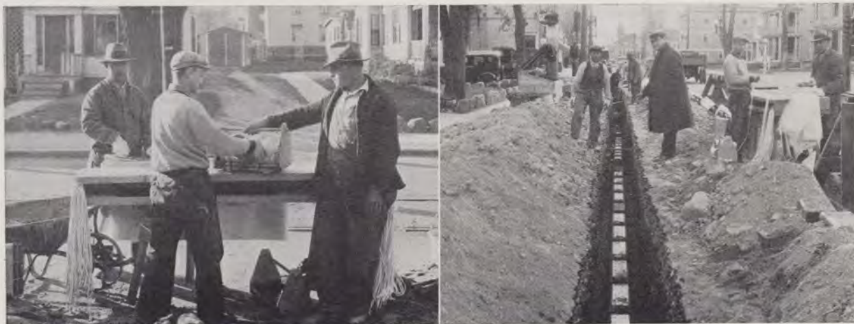
Loading carrying tray with mortar bandages for workmen in the trench. Right: Trench in N. Attleboro, showing new type of conduit construction, using mortar bandages.
