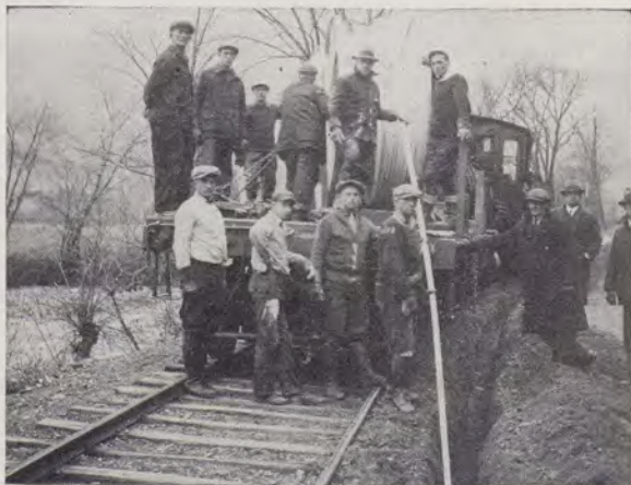
White River Valley telephone crew laying armored cable in a trench, from a train, in first job of its kind in Vermont.
