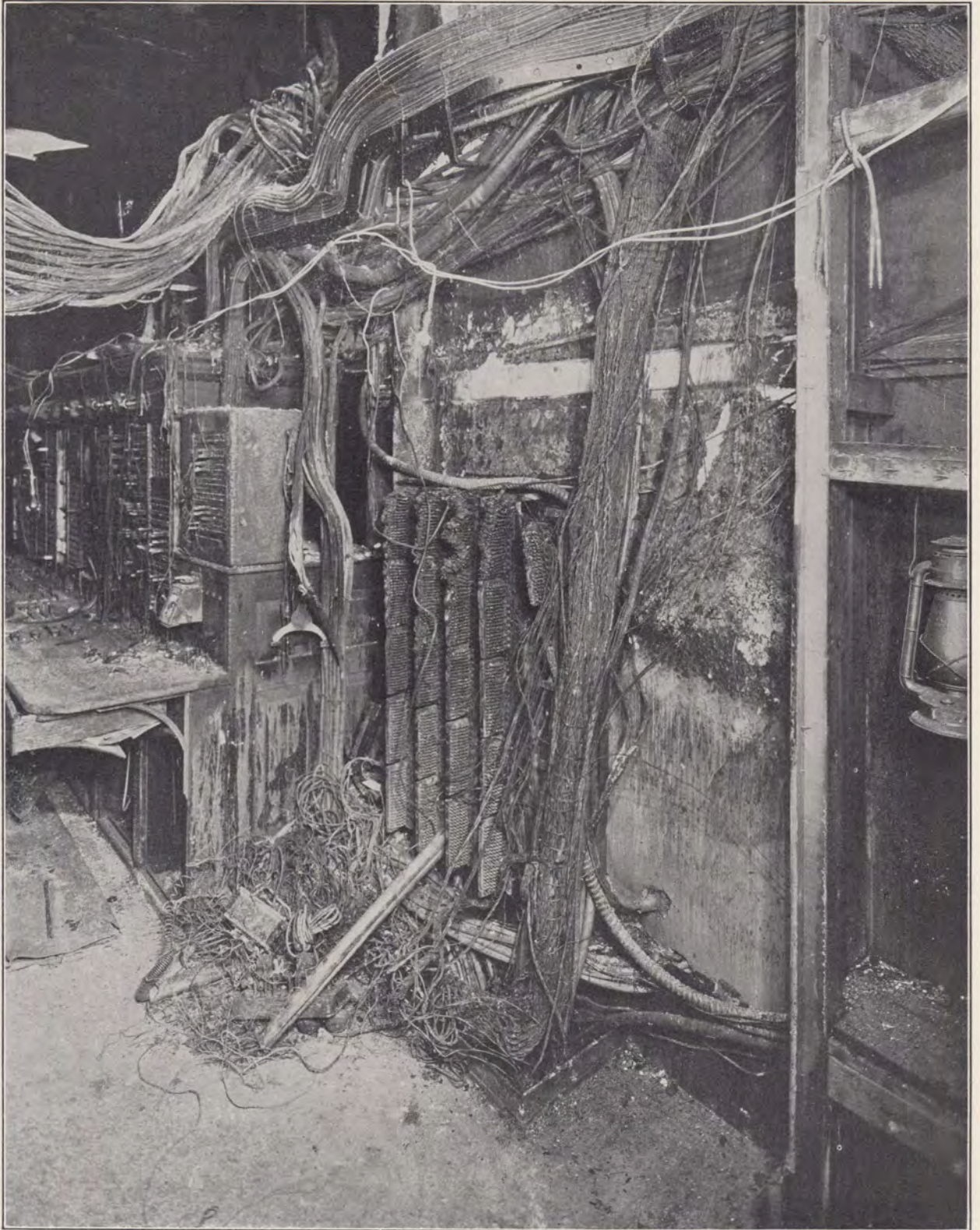
AFTER THE FIRE WAS OUT Auxiliary Toll Intermediate Distributing Frame
