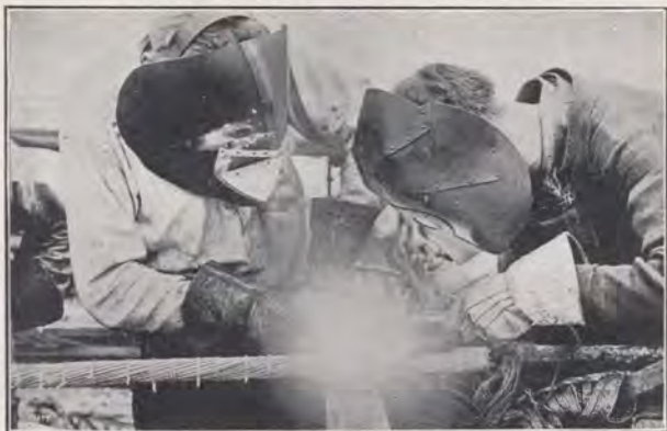
Making a splice. Welding of the armor wires by means of the electric arc. The tie wires around the splice are removed after the welding is completed
